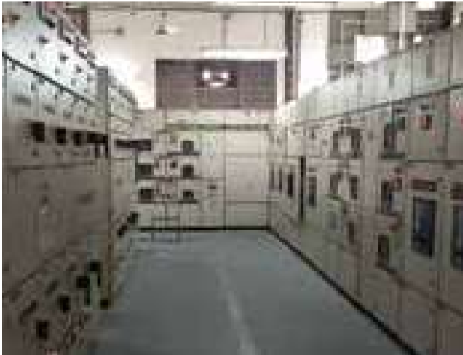
Electrical Control Room
