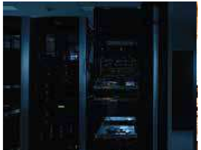
Server Room For Small Offices
